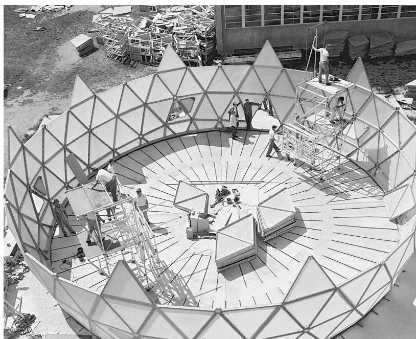
FIGURE D. A 55-ft-diameter radome being erected on the test pad between the easterly ends of Buildings B and D at Lincoln Laboratory. After the radome is complete, it can be loaded mechanically to simulate, for example, the effects of wind.
